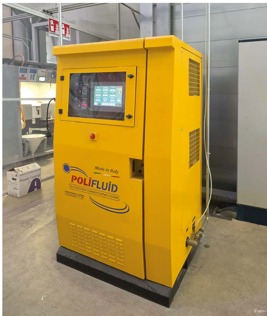
The powder coating application booths are equipped with the Polifluid system by Eurosider (Grosseto, Italy) which controls temperature and humidity of compressed air.
